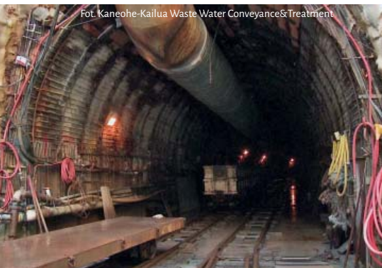
Fot. Kaneohe-Kailua Waste Water Conveyance & Treatment
